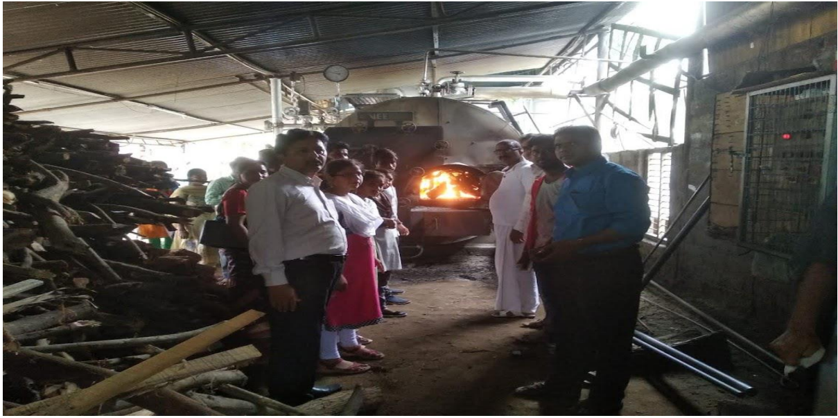
At Fire Boiler
